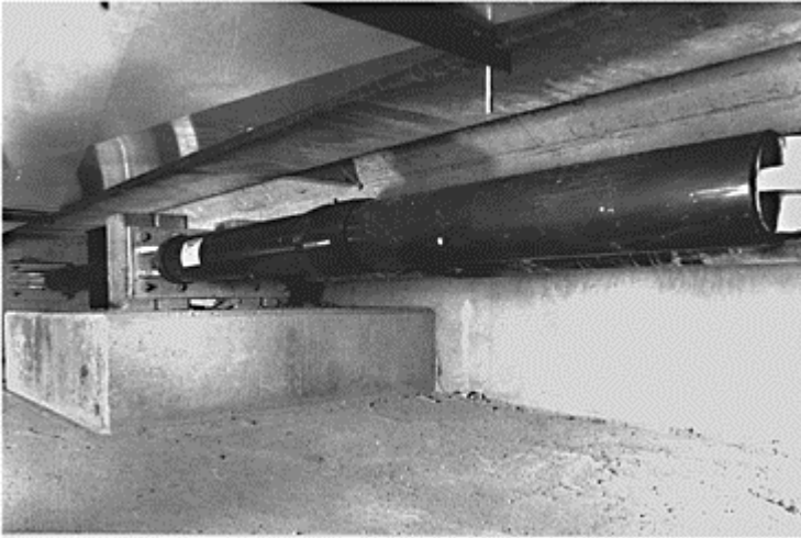
Figure 5.5.13 Lead extrusion dampers used to connect the building and the pile cap (photograph by John Bellamy, supplied by Robinson Seismic Ltd.)
