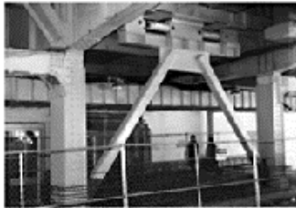
Photo of installed damper
