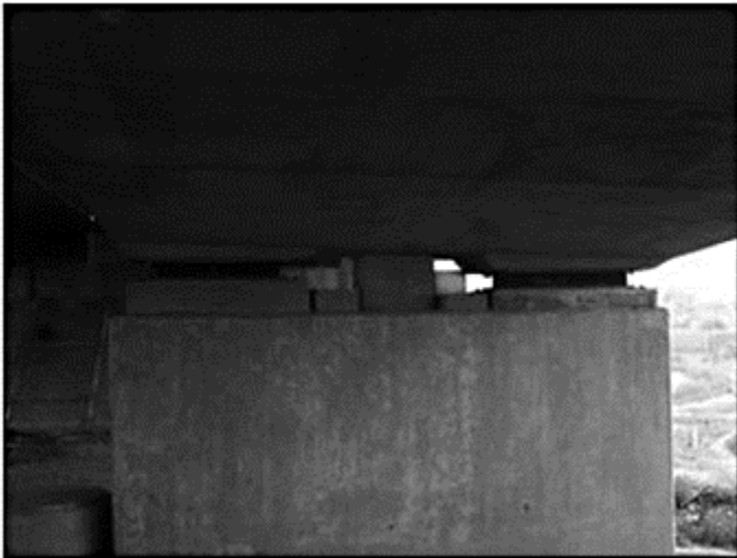
Figure 5.6.13(b) Lead-rubber bearings, Bai-Ho bridge
