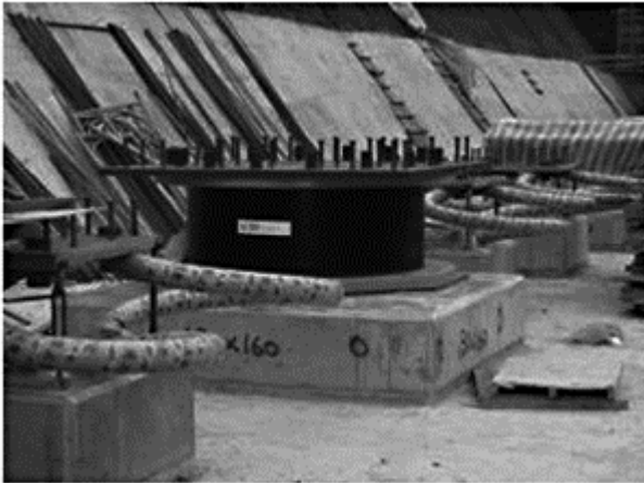
Figure 5.6.14(b) Lead-rubber isolation bearing and coil damper, Tzu-Chi Medical Center
