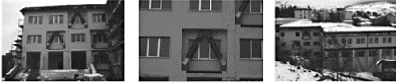
Figure 5.2.30 The “Giacomo Leopardi” school at Potenza after its retrofit by means of steel bracings provided with EPDs (photographs by the courtesy of Prof. M.Dolce and Tis, Rome, Italy)
