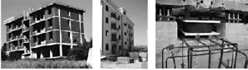
Figure 5.2.29 One of the Solarino residential buildings before and after (2004) retrofit with SI; installation of a HDRB during retrofit (photographs by the courtesy of Prof. G.Oliveto and Fip Industriale, Selvazzano, Padua, Italy)
