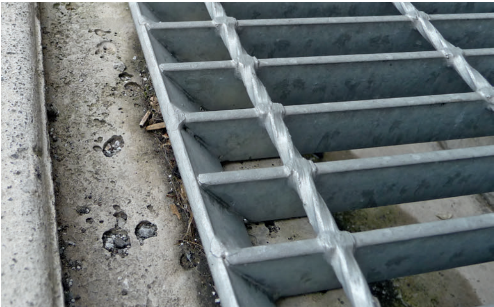
8.16 45 degree sliding surfaces between concrete paving and a steel grating cover plate, Wellington, New Zealand
