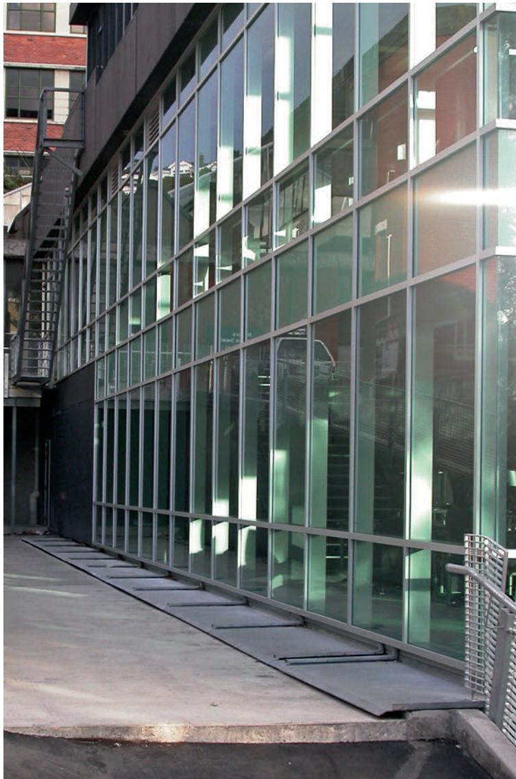
7.19 Galvanized steel plates cover the rattle space between retaining wall and isolated superstructure
