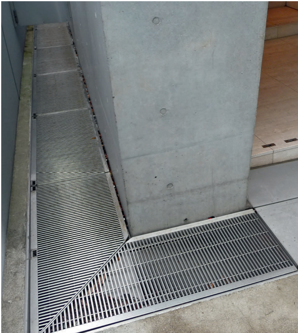
8.22 A steel grill cover plate where drainage is integrated with a moat space, Tokyo, Japan
