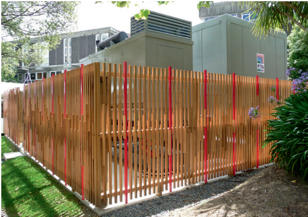
5.15 A 3-D seismically isolated back-up data centre, Victoria University of Wellington. The main module is behind the self-contained UPS generator to the left
