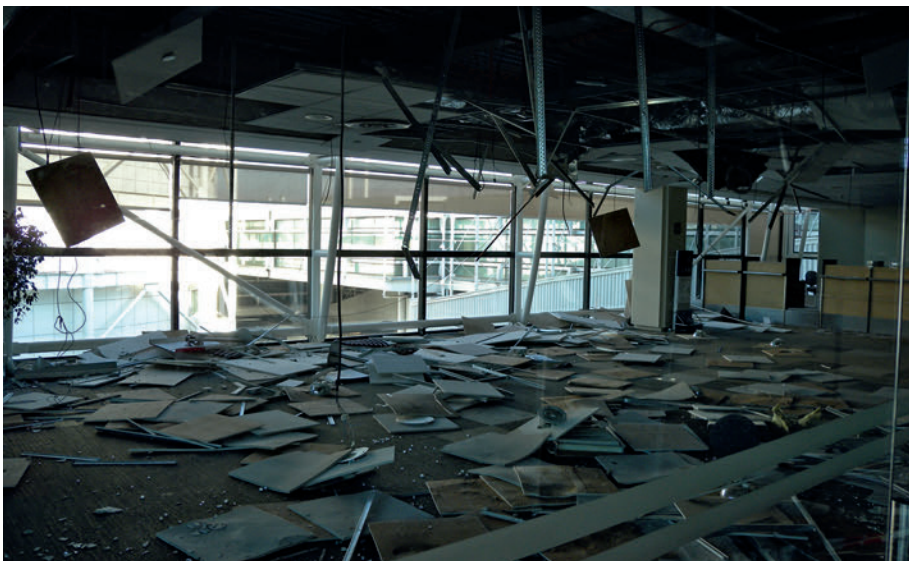
5.8 Non-structural damage to a suspended ceiling at the Santiago International Airport terminal building after the 27 February 2010 Chile earthquake
