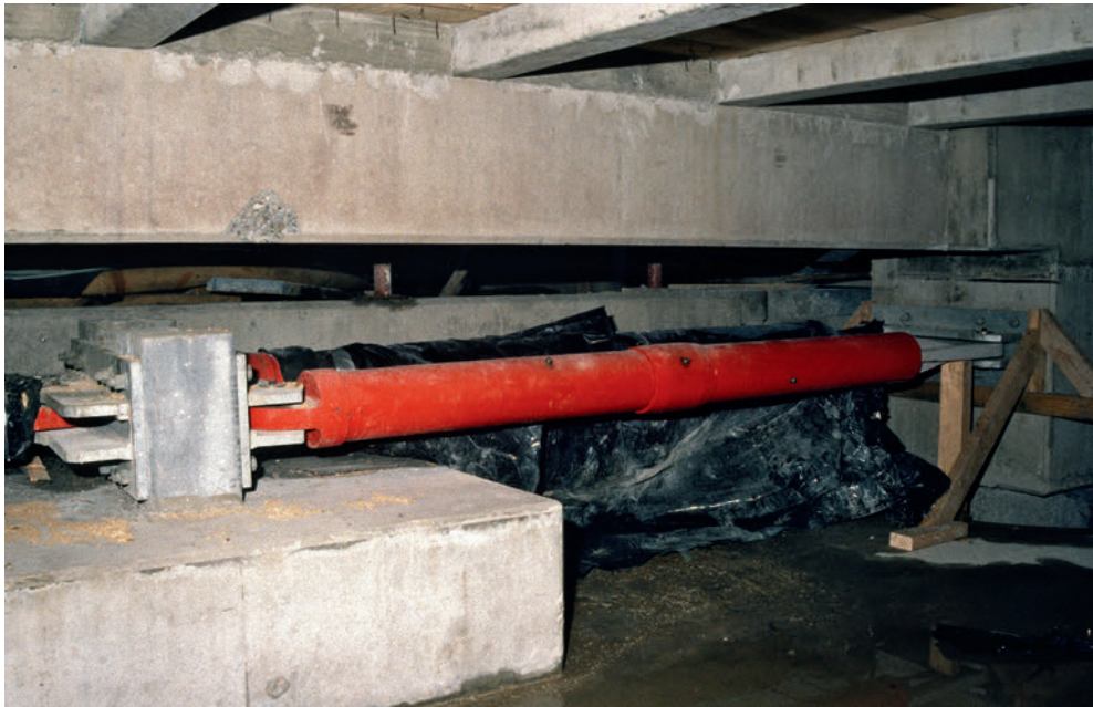
3.7 A lead-extrusion damper in the basement of the Wellington Central Police Station
