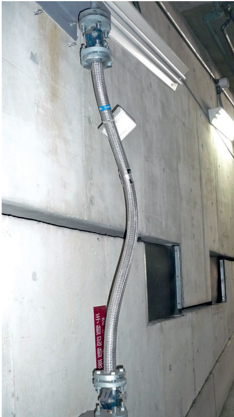
8.35 A flexible pipe crossing an isolation plane, Tokyo, Japan
