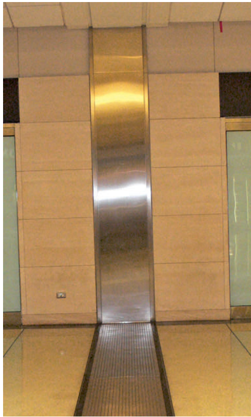
8.23 A visible surface (and wall) mounted interior cover plate, San Francisco, USA
