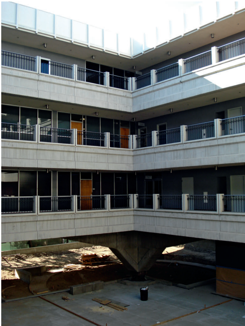
2.10 Glendale City Hall, Glendale, USA. The interior courtyard showing one of the isolators used to retrofit the original 1927 building
