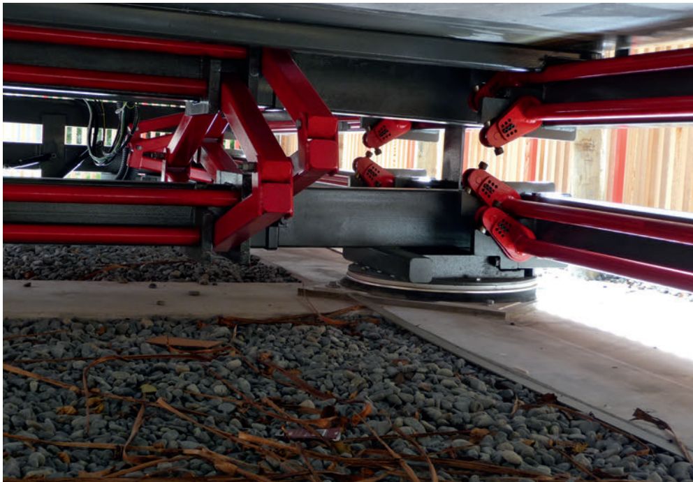
5.16 A LoGlider bearing supporting the platform. The red mechanical components provide vertical isolation
