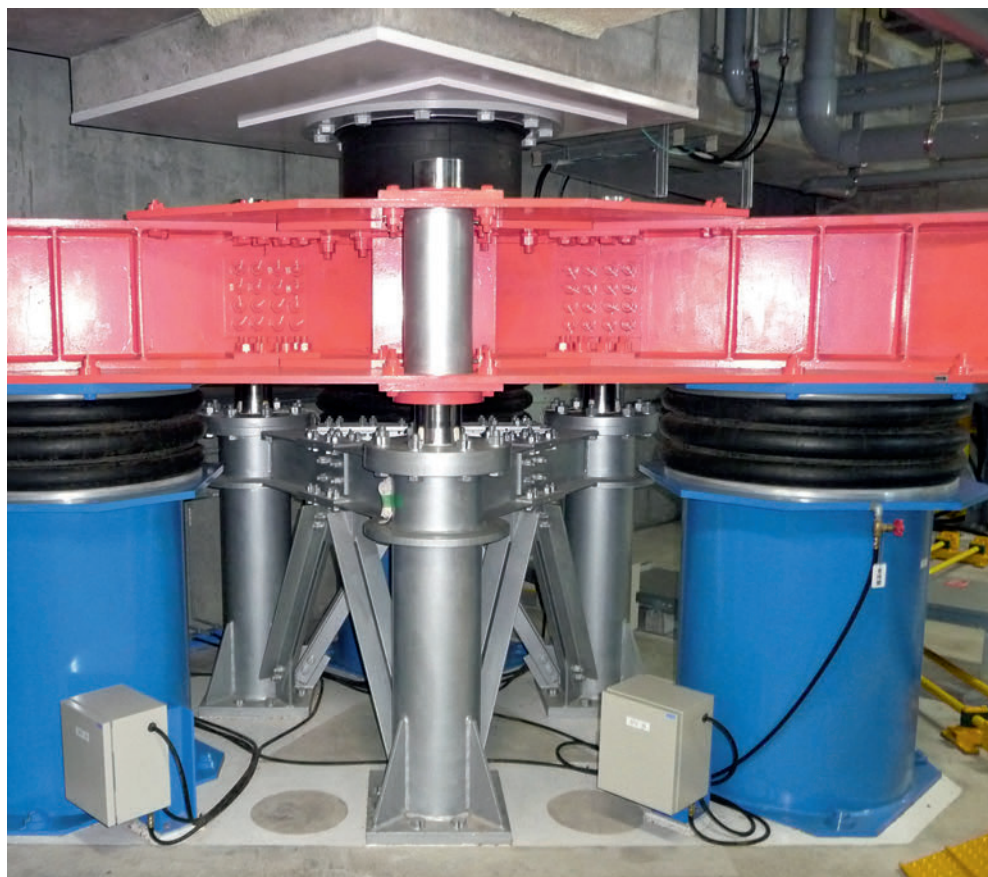
5.12 The 3-D isolation system of Chisuikan. Located in a basement, vertical isolation is achieved through the air-springs atop three blue cylinders and silver-coloured dampers. The bearing above the red beams provides horizontal isolation
