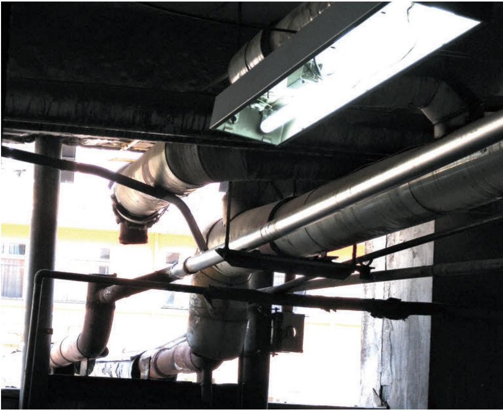
5.9 Damage to ceiling mounted mechanical services at the Santiago International Airport terminal building after the 27 February 2010 Chile earthquake
