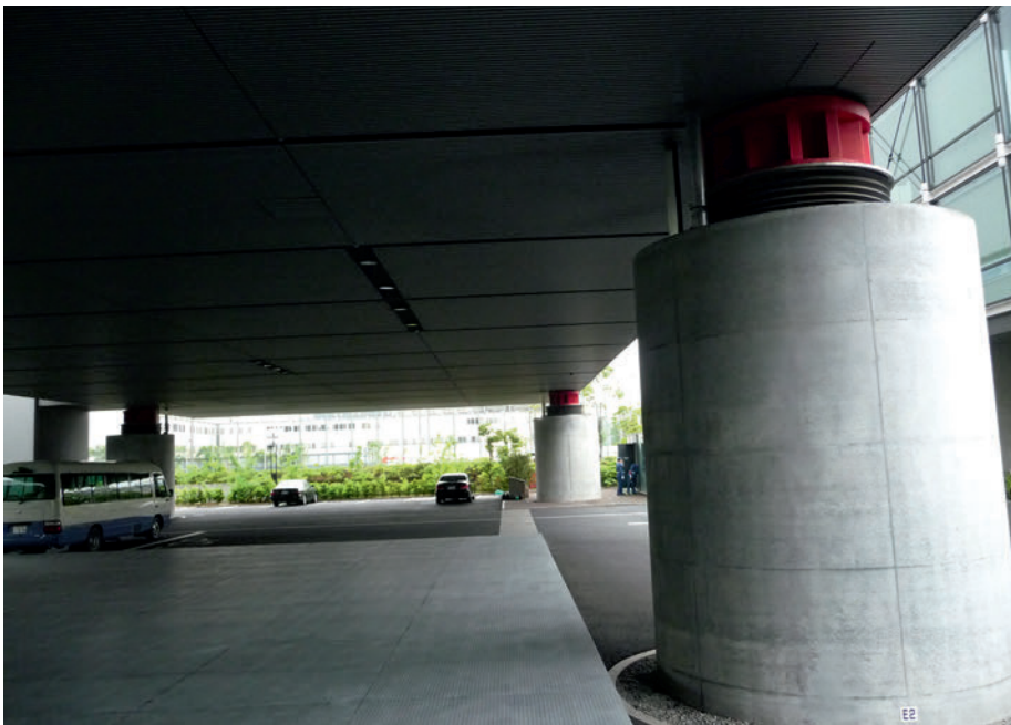
6.6 Shimizu Institute of Technology, Tokyo, Japan. Some of the piers and isolators supporting the main building
